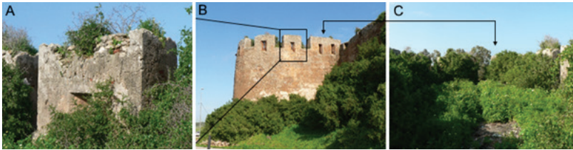
Fig. 3. Vegetation colonizing the ashlar enclosure adjoining the “U” shaped Porto–bastion (B) as well as its walls inside (A) and the floor (C) losing all reading of the site
